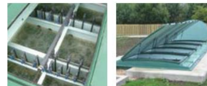
Internal air diffusers (left) and large gas strut lids (right)
